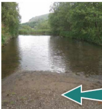
Silting at Parc Cwm Darran Lake
